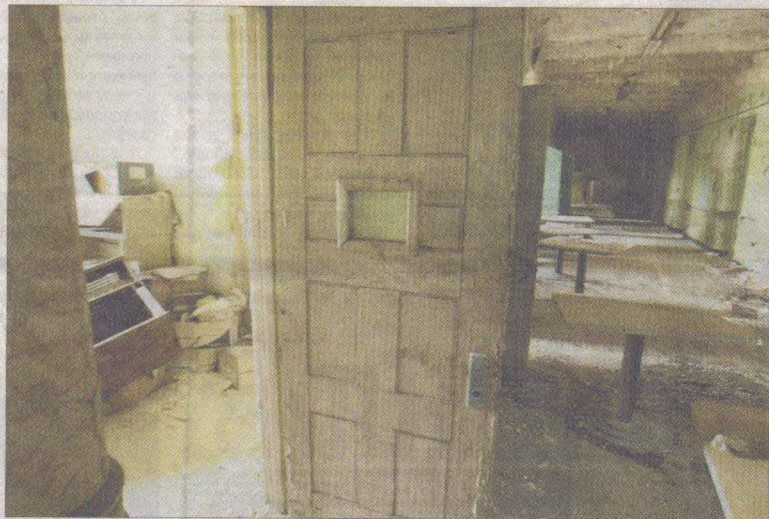
This was once a patients ward in the old hospital building. Preservationists fear the cash-strapped state could sell Greystone to a developer.
